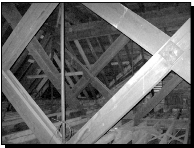
The complicated wood truss system under the roof of the courthouse has never been documented or analyzed
